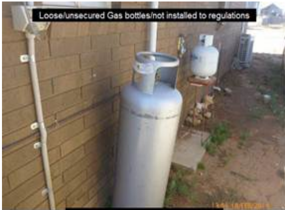
Gas cylinders unsecured – potential for injury (2013)
