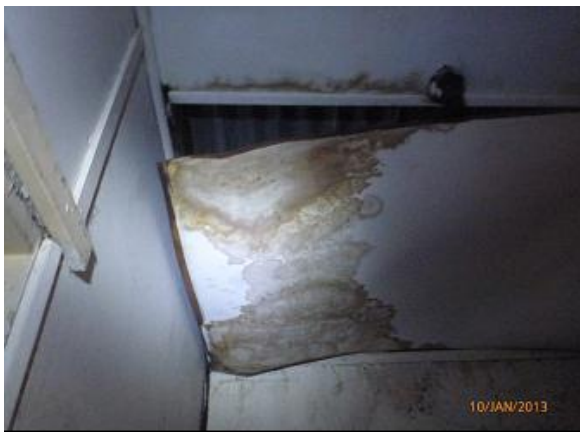
Ceilings sagged, water damaged (2013)
