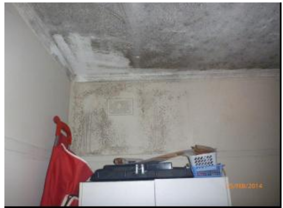
Mould on ceilings throughout house (2014)
