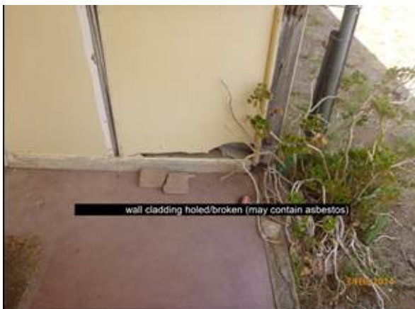
Deteriorated wall cladding may contain asbestos (2014)
