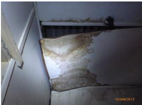
Ceilings sagged, water damaged (2013)
