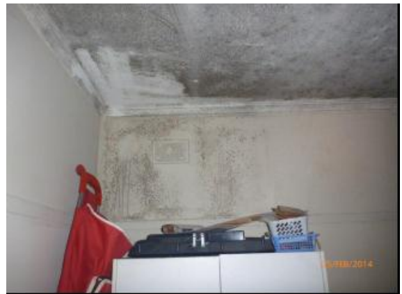
Mould on ceilings throughout house (2014)
